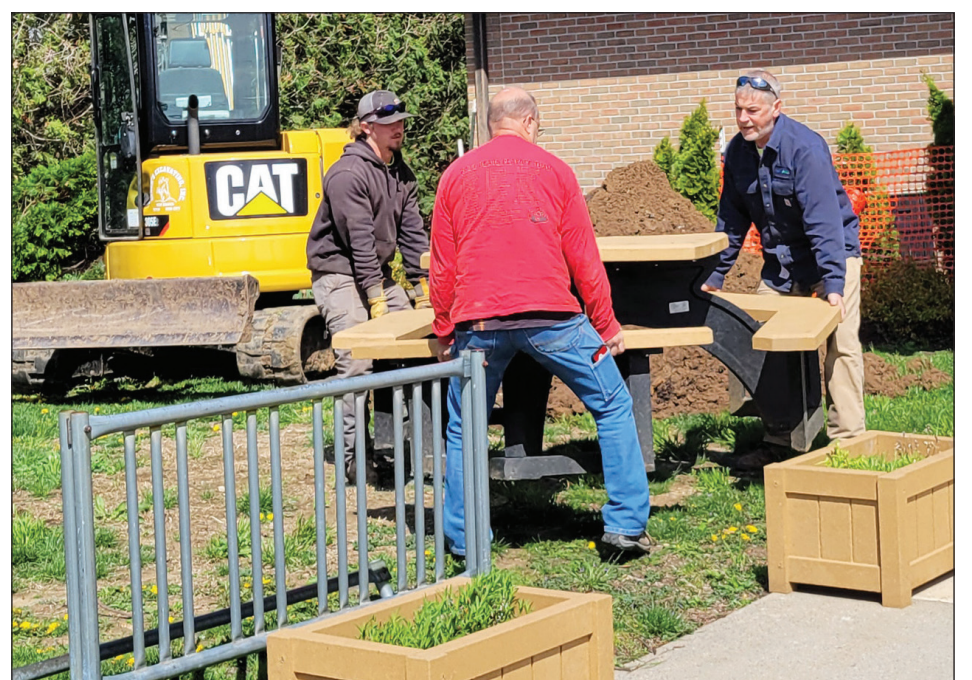
Mayor Roger Laughlin (center) helps Lynch's Excavation workers move a picnic table on Friday as Lynch's digs up the soft ground before refilling the hole and compacting it. Gregory R. Norfleet/West Branch Times
