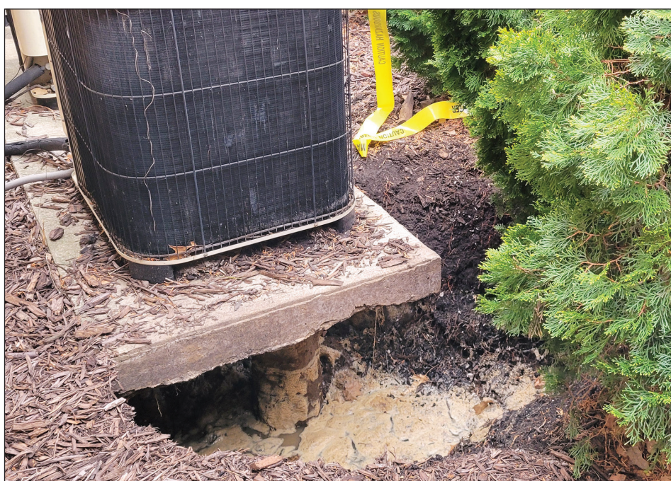
More than a week after the sinkhole was discovered, this picture shows the site on April 17. Water in the bottom of the hole made it difficult to measure the depth, but the hole is about three feet wide. Gregory R. Norfleet/West Branch Times
